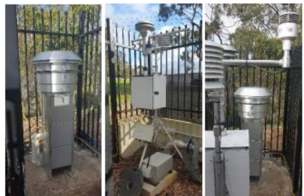
Images: Air quality monitoring equipment
