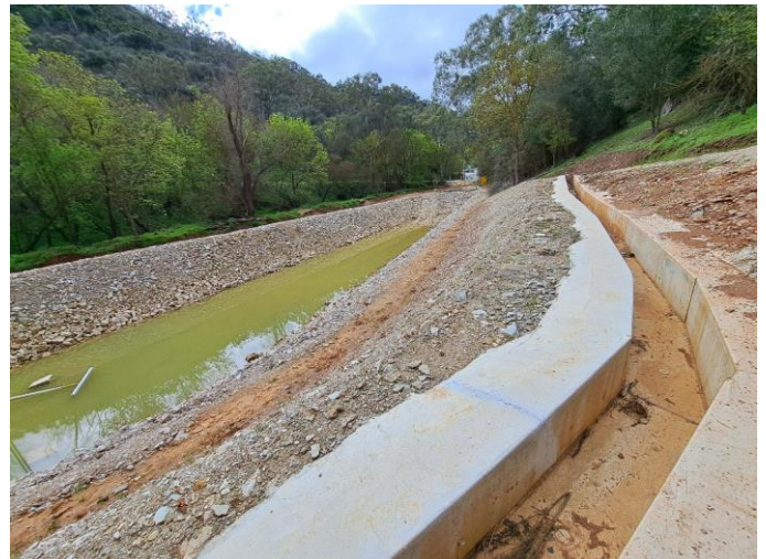
Image: New SB2A facing east – concrete drain for clean water diversion (surface water from the hill)
