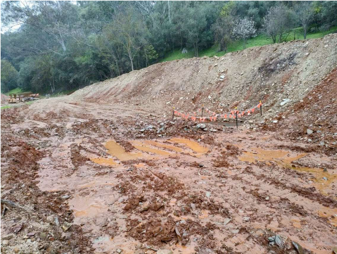
Figure 3. Current progress of the sediment basin (August 29 2022). Note the sump cordoned by flagging tape.
