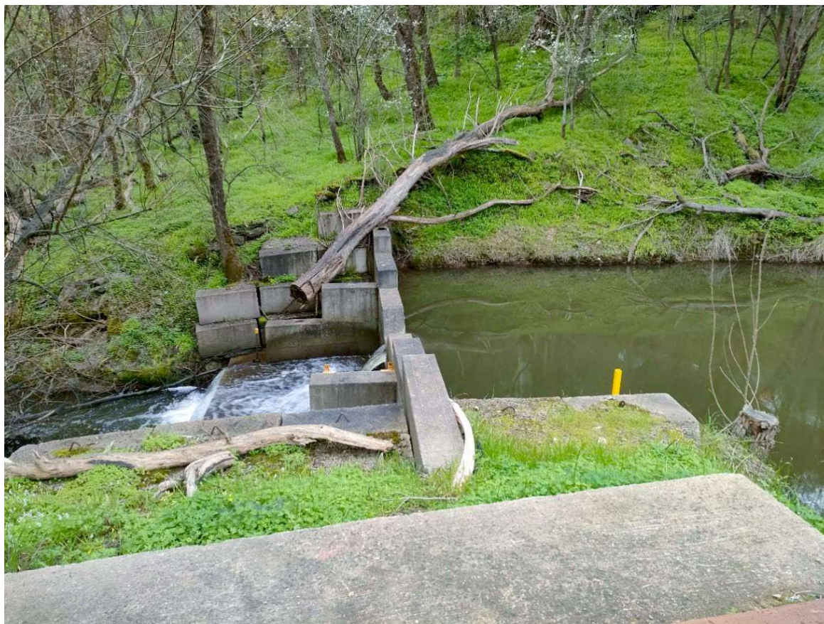
Figure 5. V-notch weir constructed in 3 rd Creek, approximately 120 m downstream of the sediment basin.
