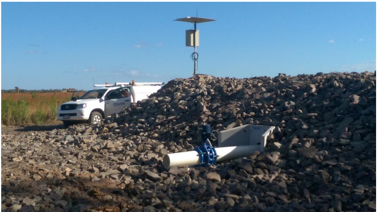
Image 4. Iqad monitoring system with auto controlled shutoff valve on outlet.
