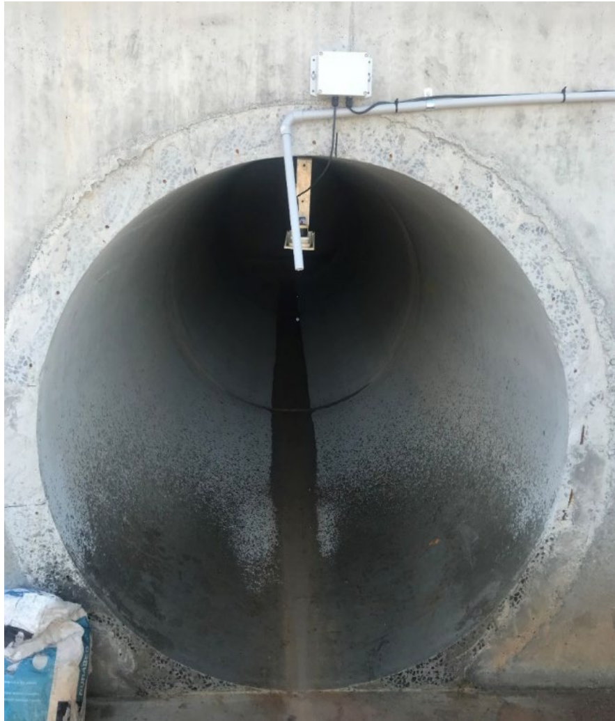
Mounted Ultrasonic Sensor and coagulant discharge line above flow of water
